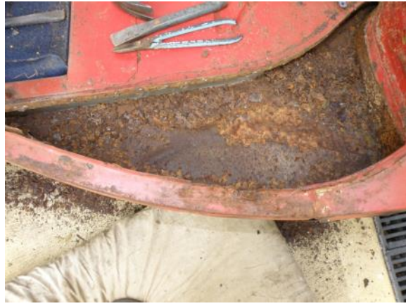
Figure 6. Showing rust on the bottom triangle.
